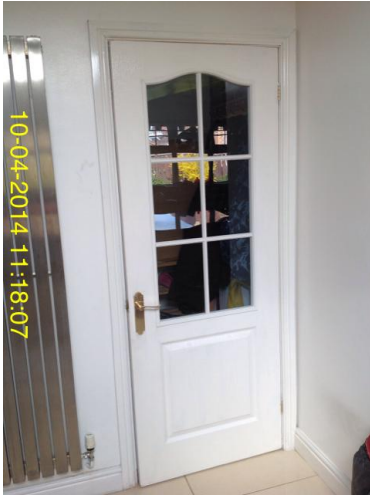
Utility Room - Door and Frame
