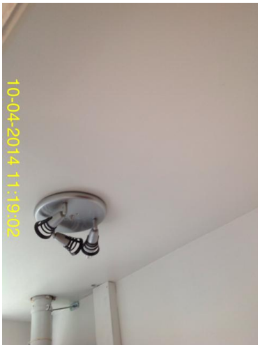
Utility Room - Fittings
