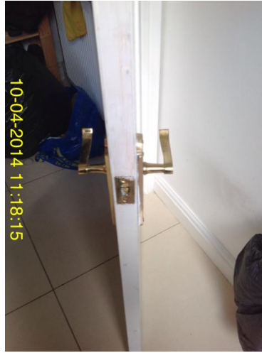
Utility Room - Door and Frame
