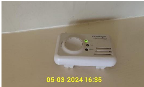
6.1.1 - CO Alarms - condition
